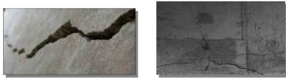
Figure 1: (Left) Crack on road (Right) Crack on building wall
