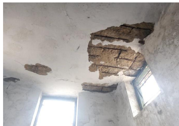
Figure 1 Spalled ceiling at QTR No. –19-24, Shastri Nagar, Patna
