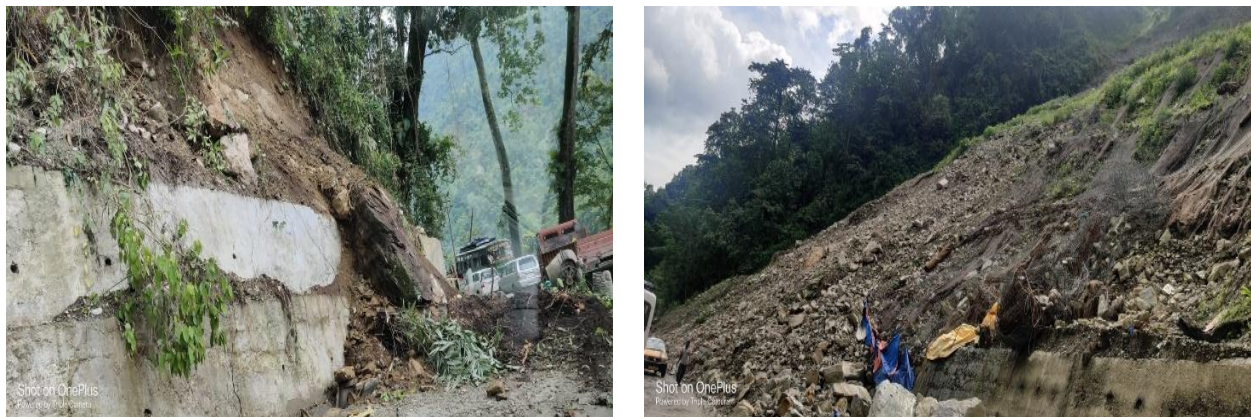
Figure 2 Slope failures at Kalijhora on Sikkim Highway, in Indian Himalayan (images by author)
