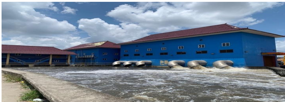
Figure 7 Gravity outlet and pumping system at the Bendung river mouth
